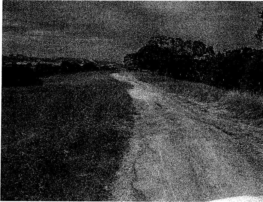
Photo 4. View north of the waterline route along the outer edge of blue oak woodland habitat. Station 35+00 to 30+00.
